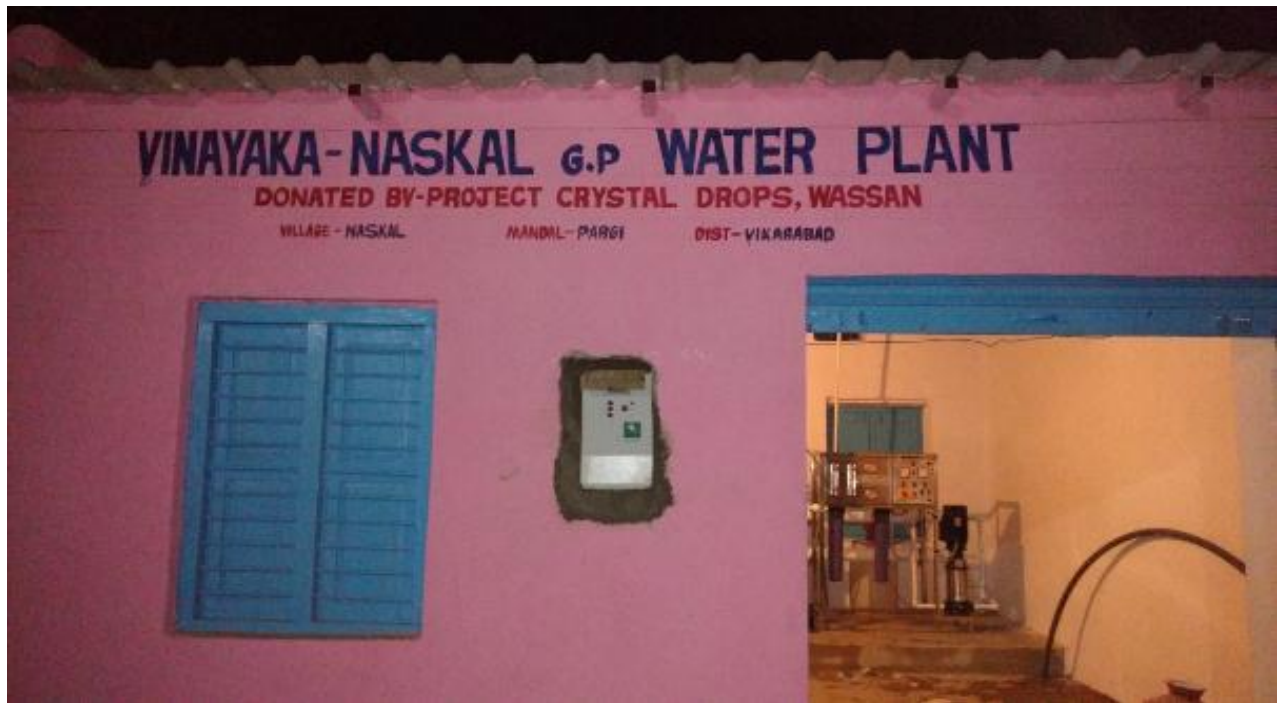
New RO plant installed in Naskal – 2017
